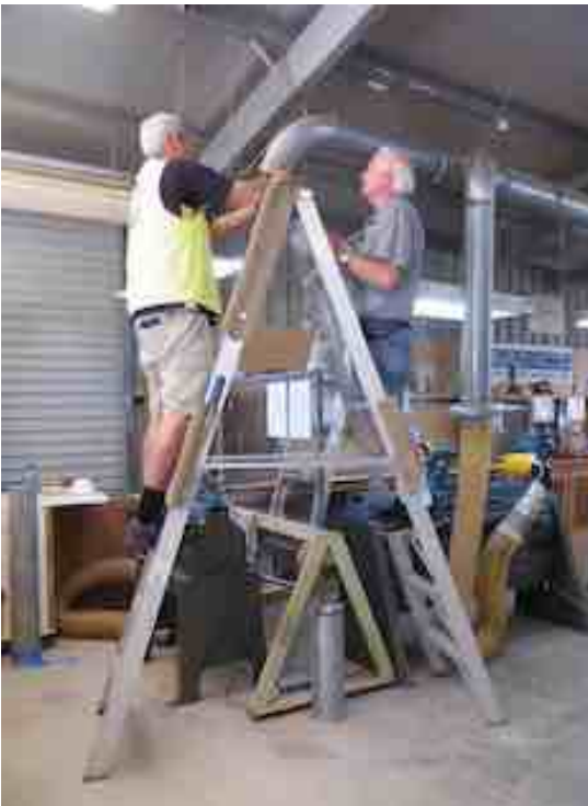
Warrick King and Daryl Stephenson improving the ducting system to the lathe area
